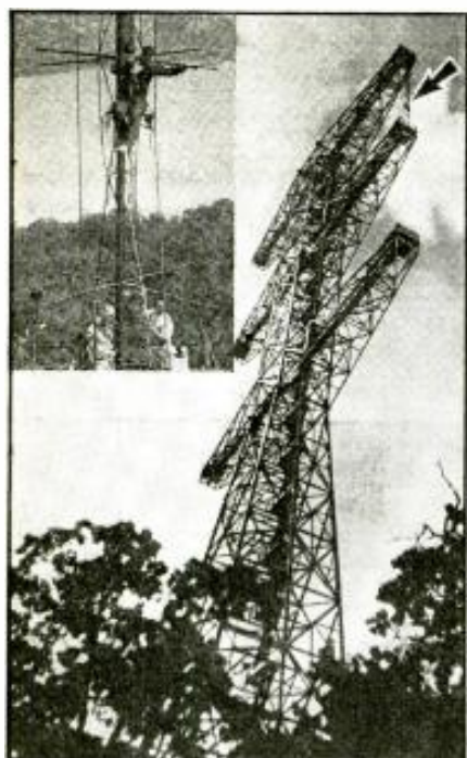
(Inset Photo—Norman Monroe, Alpino Police.) The adjustment of this antenna (shown during the early stages of its construction), located at Alpine, N. J., proved to be the most difficult part of the whole construction. For a period of 2 months last summer Major Armstrong sat in a boatswain's chair (see inset) several hours a day 400 ft. up regulating the transmission lines. "As this had to be done with the power on, the combination of dodging the high voltage and the frequent thunder storms made the day's work always an interesting one," Major Armstrong said.
